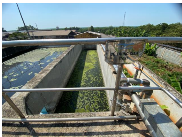
Bể trung gian
